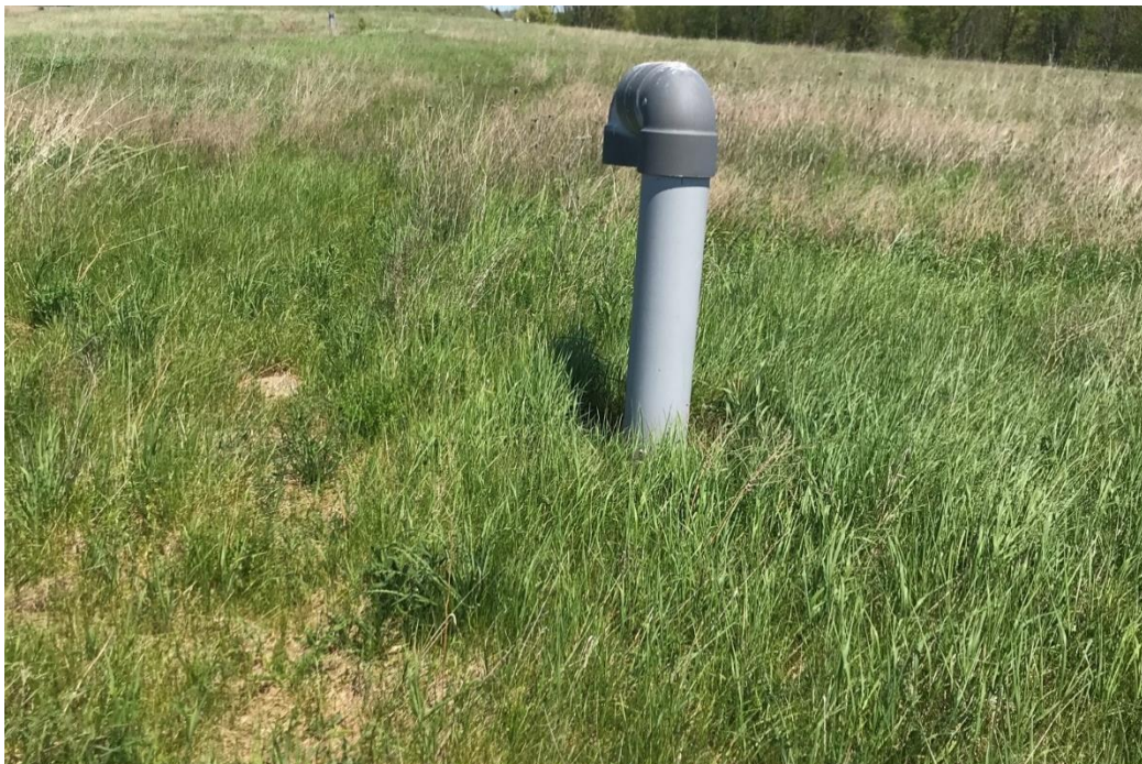
Photo 6: View of methane vent (May 2021).
