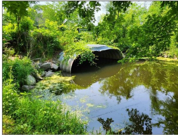
North elevation (deformation at culvert obvert)
